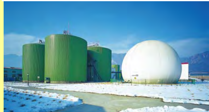
Yanqing 2 MW Biomass Gas Project in BJ
