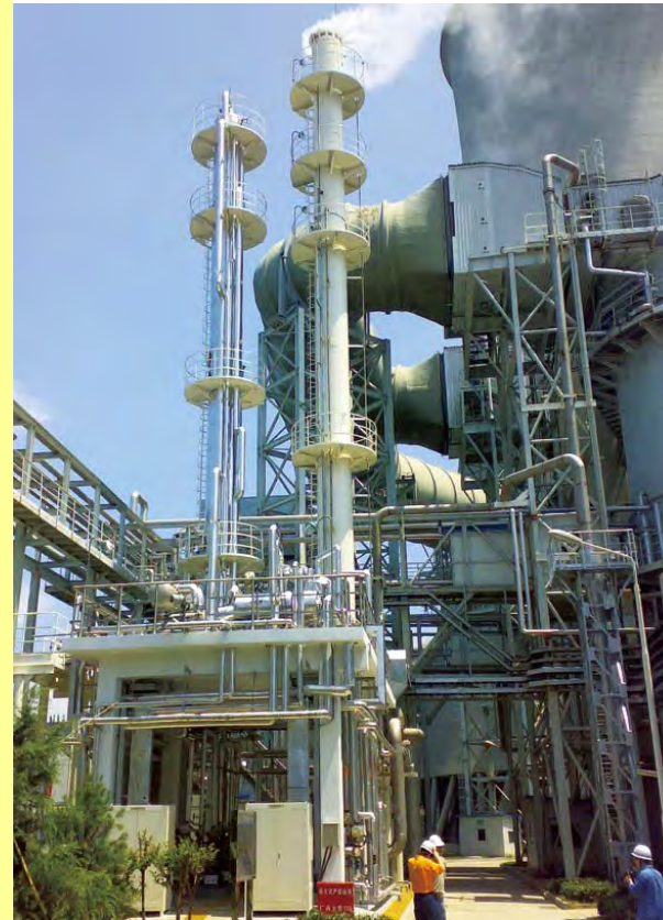
120,000 t/a CO 2 Capture Project in Shanghai
